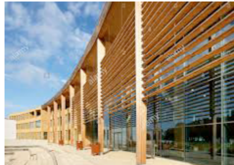
External Shading External shading devices can be incorporated to prevent excessive internal solar gains and avoid overheating
